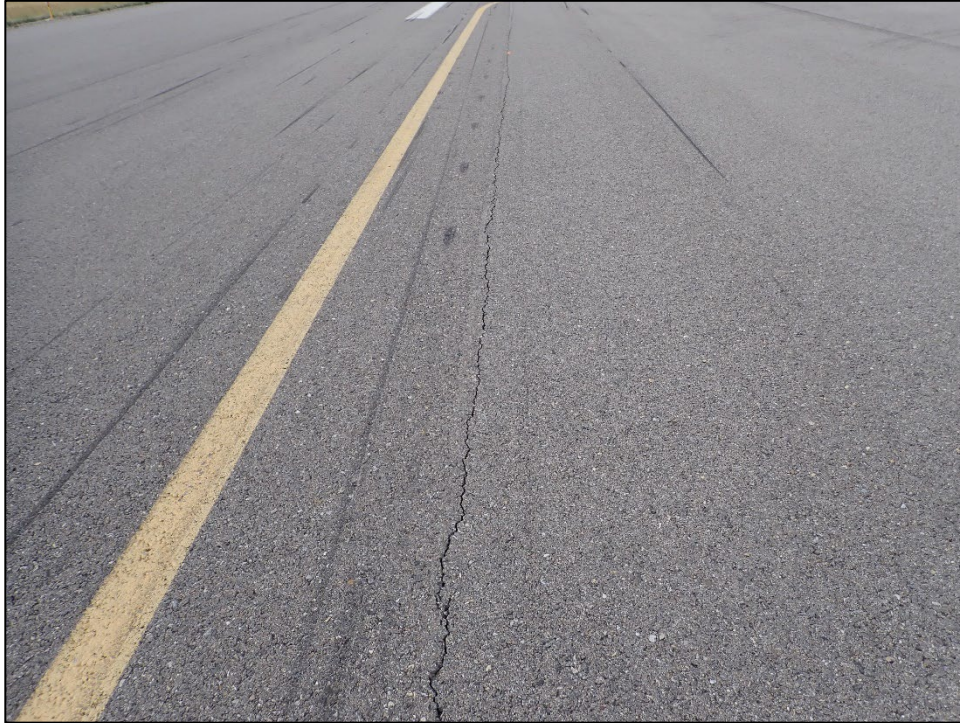
RW12-01-13: L&T Cracking
