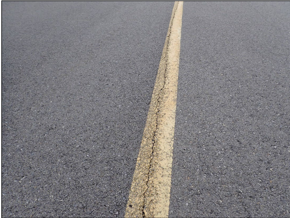
TW-01-04: L&T Cracking
