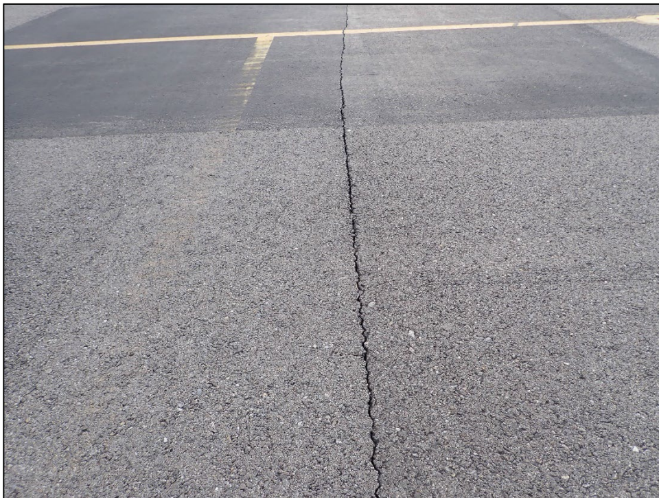
AP-02-11: L&T Cracking
