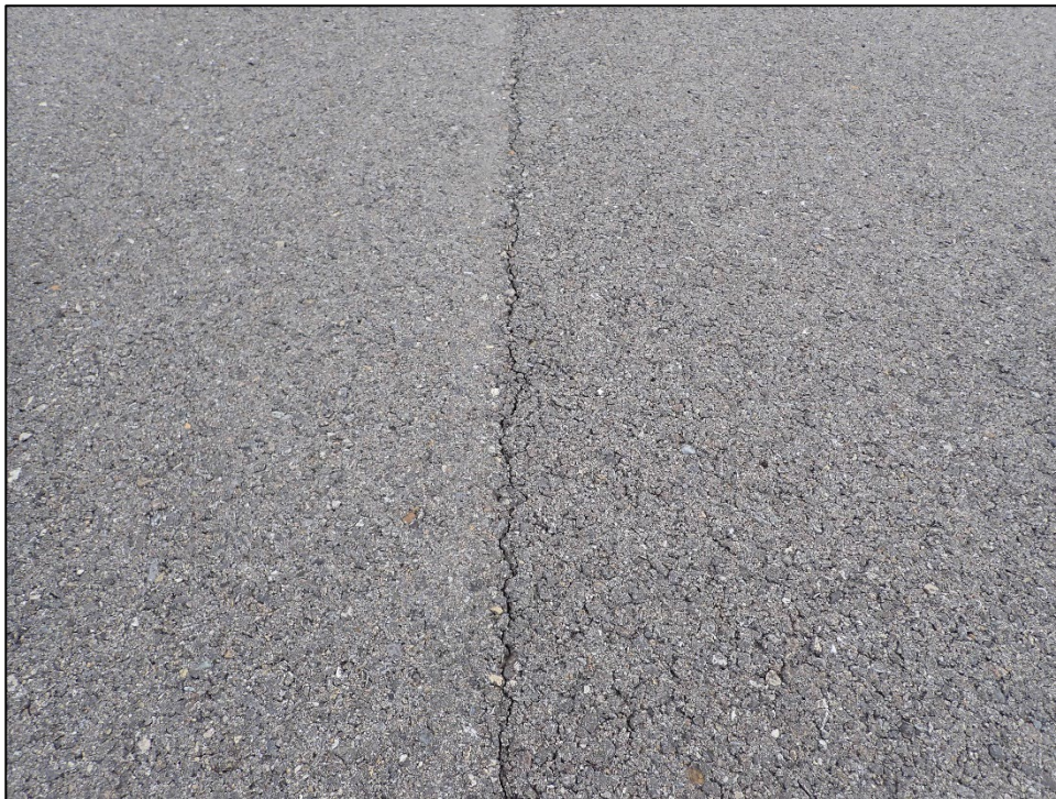
RW12-01-44: L&T Cracking
