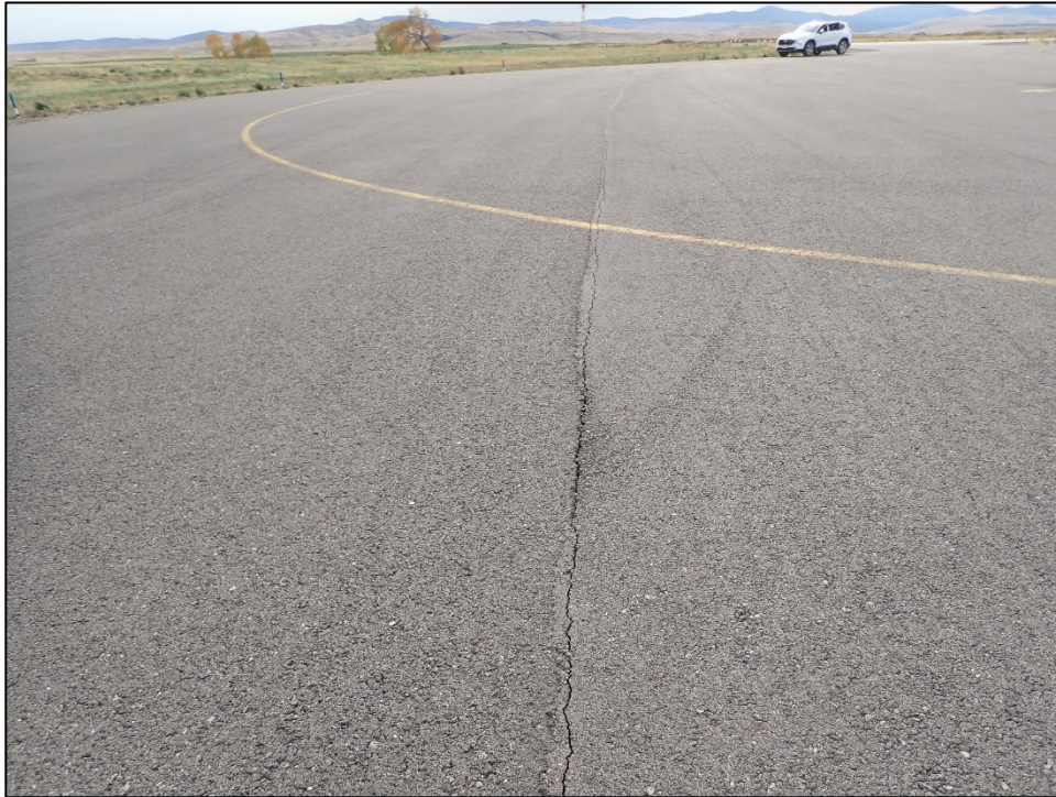
AP-02-01: L&T Cracking
